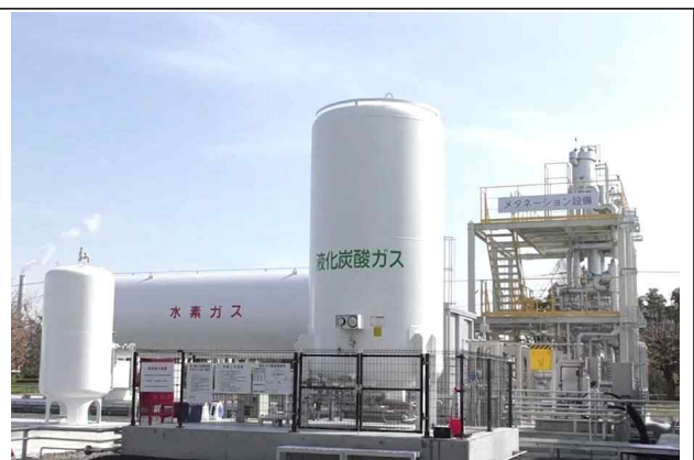
▲ Hydrogen tanks and CO 2 tanks
